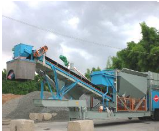
Gambar II.6 Mobile Batching Plant PT SCG Readymix Indonesia
